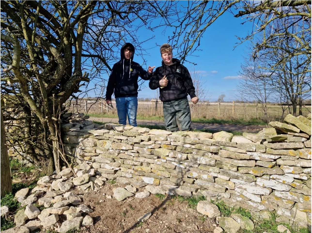
Students from The Cotswold School learning how to build a dry-stone wall © Jonty Brunyee
