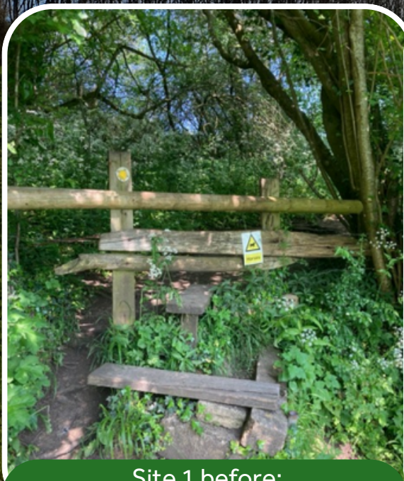
Site 1 before: Unstable steps, degraded stile, overgrown
